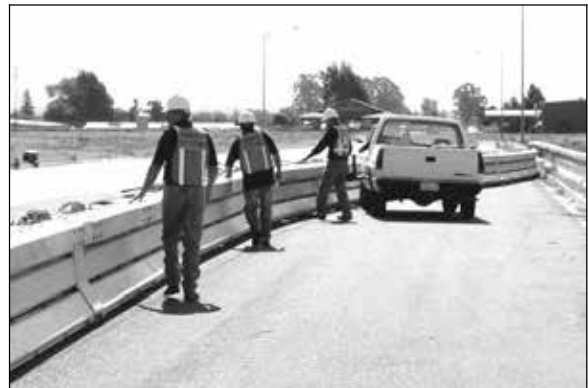
Figure 20. As the wall is being repositioned personnel lower each section at its final deployment or storage position.
